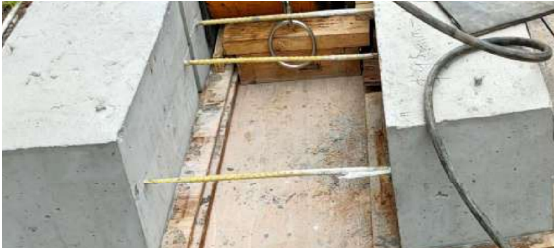
FRP leg / concrete block view
